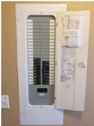
200 amp Electric Service on Main Floor (Standard Dropped to Basement)
